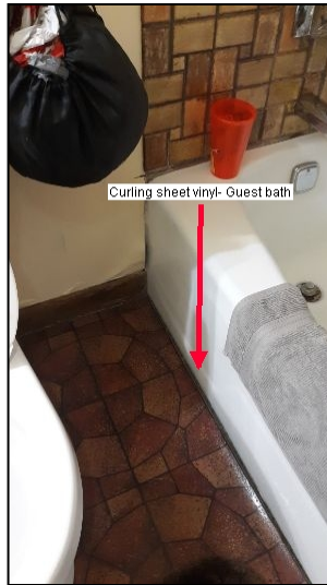
Defect: Sheet vinyl is curling up near the bathtub.
