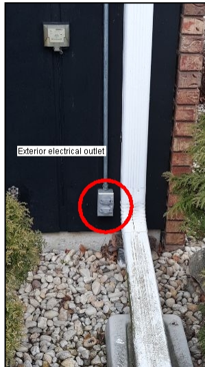
Exterior outlets were not GFCI protected.
