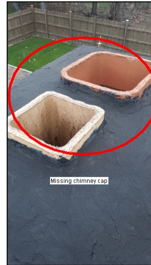
Defect: The chimney is missing a flue cap.
